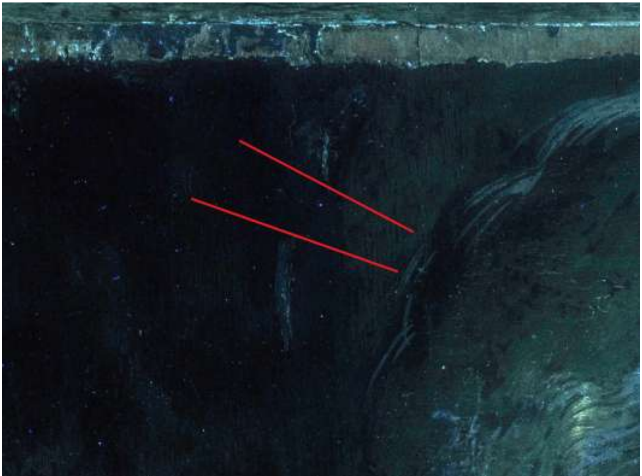
Fig. 13: The red lines indicate the point of interruption caused by a past restoration.
